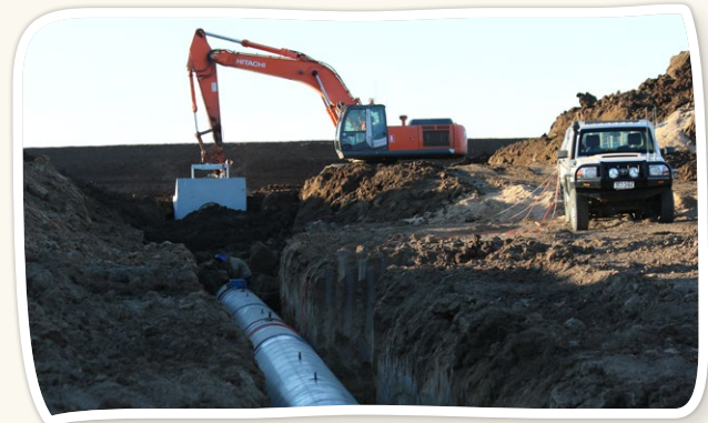
The scale of earthworks to install 220 metres of pipe was impressive, and created an inverted siphon beneath Brayland Lagoon.
